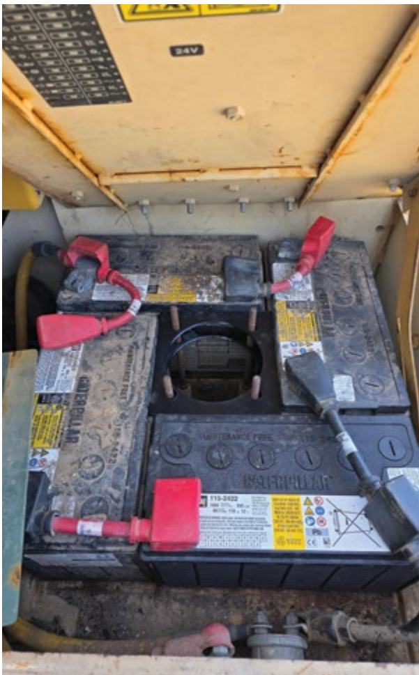
Figure 1: D7 Dozer batteries with retainer missing (Photo by 1LT John Douglas)
