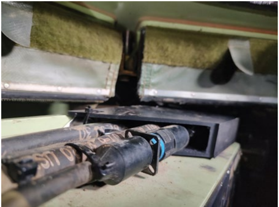
Figure 6. Image of CAN bus cables with 3D printed bracket installed. (Image by SFC Donald Fadel)
